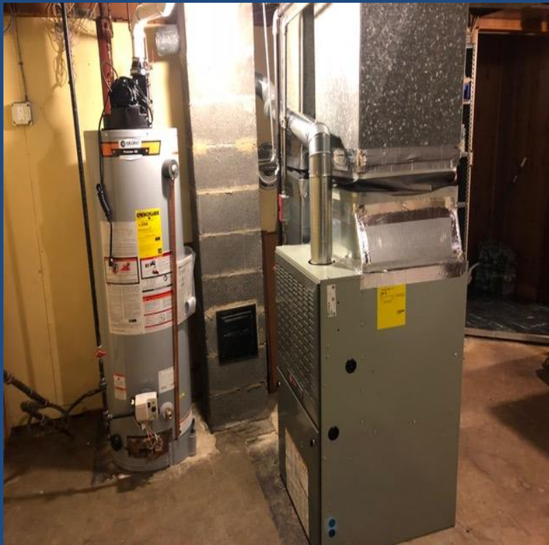
Completed heating unit and water heater.
